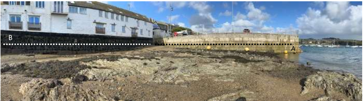
Figure 2: Site Overview – Seawall A (black dotted line), Seawall B (white dotted line)
